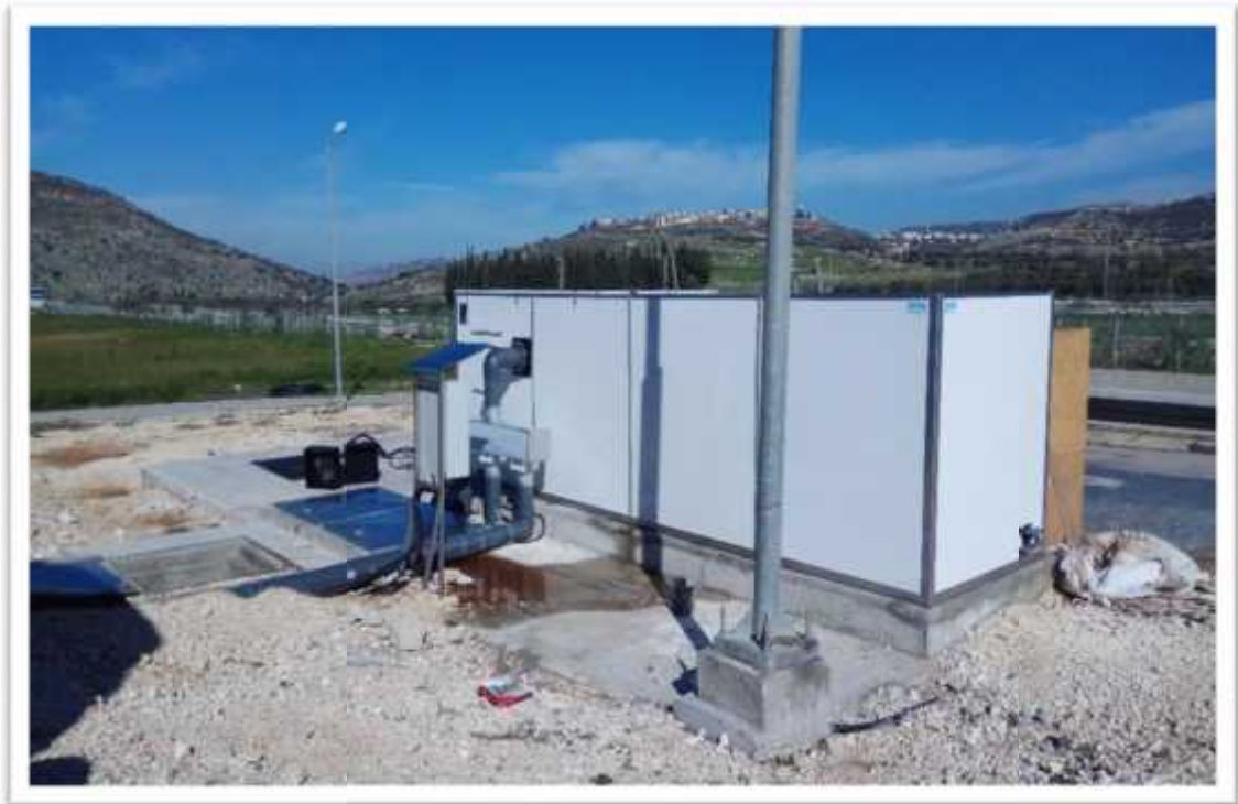
Figure (10): Odor control (bio filter to treat the gases of the primary thickener and Zibar storage tanks)
