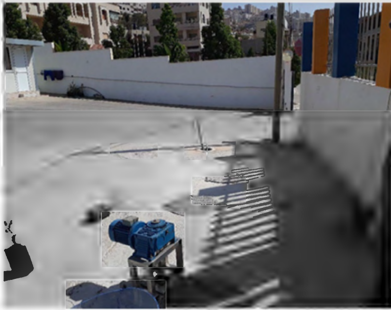
Figure 11: Pre-Treatment Unit at Dana Veterinary Factory
