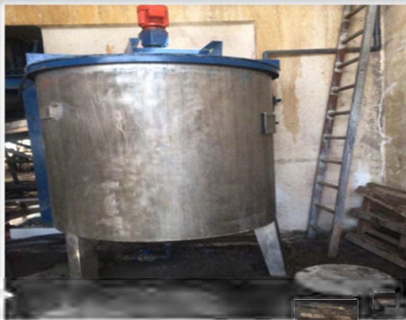
Figure 12: Additional pretreatment unit
