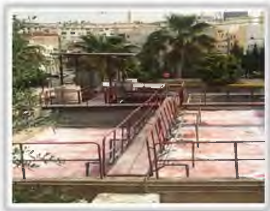
Figure 15: pretreatment units for pharmaceutical factory in Jordan
