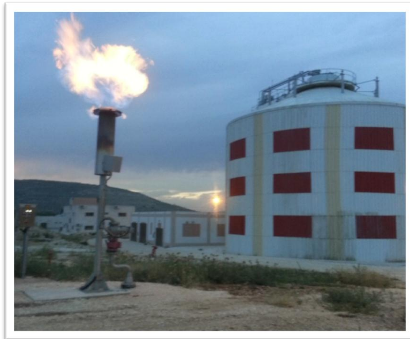
Figure (6): Digester tank in Nablus West WWTP with the gas flare
