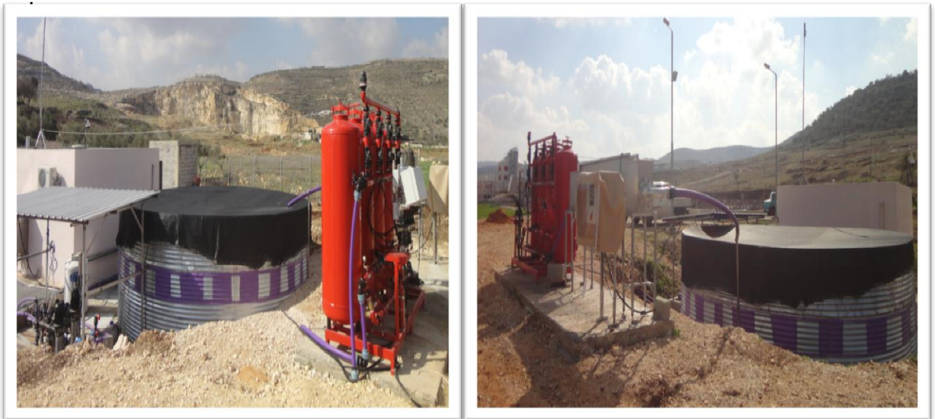
Figure (15): Sand filtration and ultraviolet disinfection units
