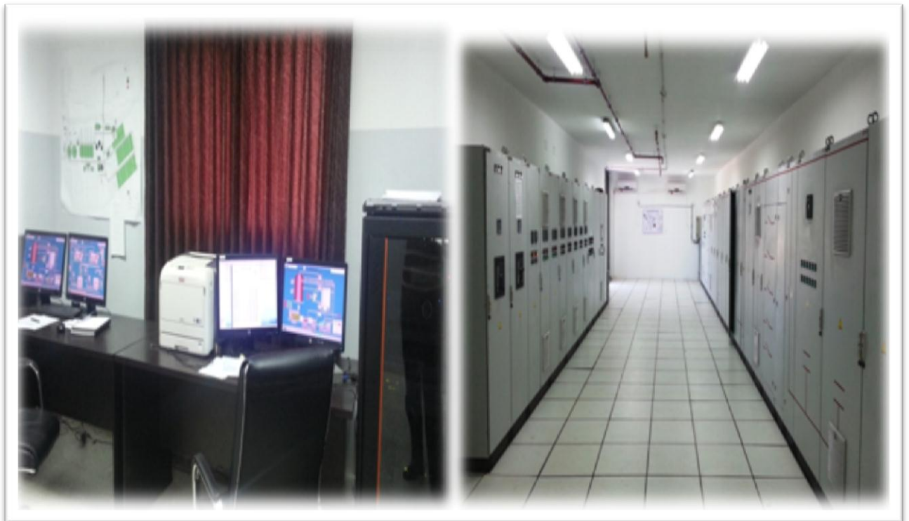
Figure (8): Nablus WWTP SCADA system
