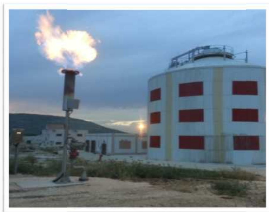
Figure (6): Digester tank in Nablus West WWTP with the gas flare
