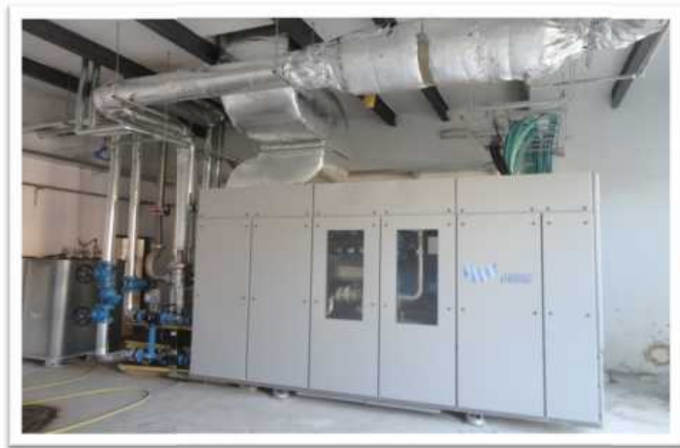
Figure (22): Nablus West CHP engine.
