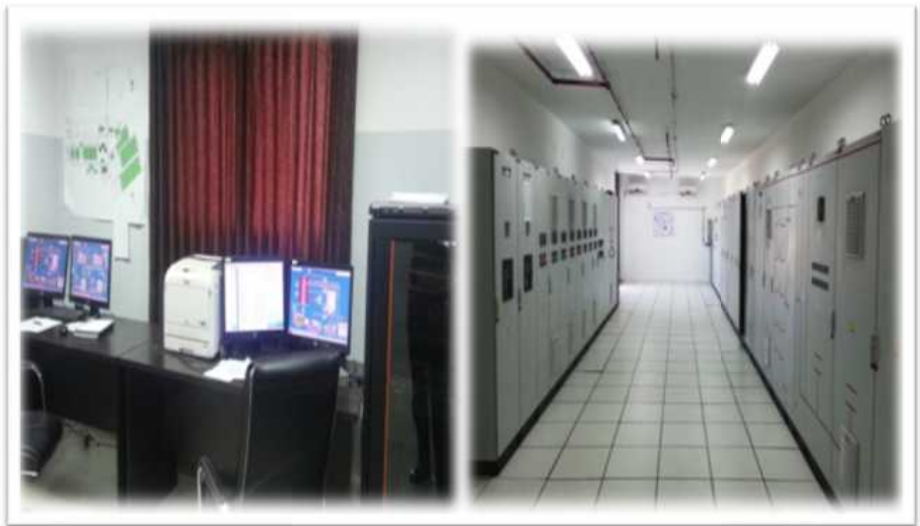
Figure (13): Nablus WWTP SCADA system
