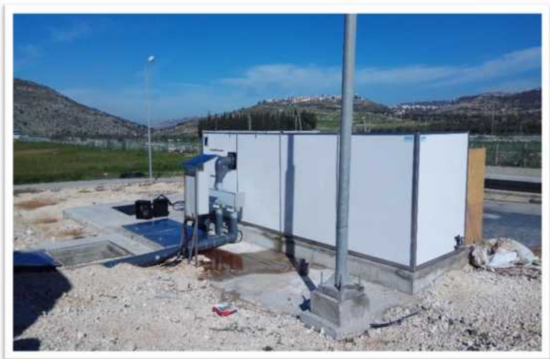
Figure (10): Odor control (bio filter to treat the gases of the primary thickener and Zibar storage tanks)
