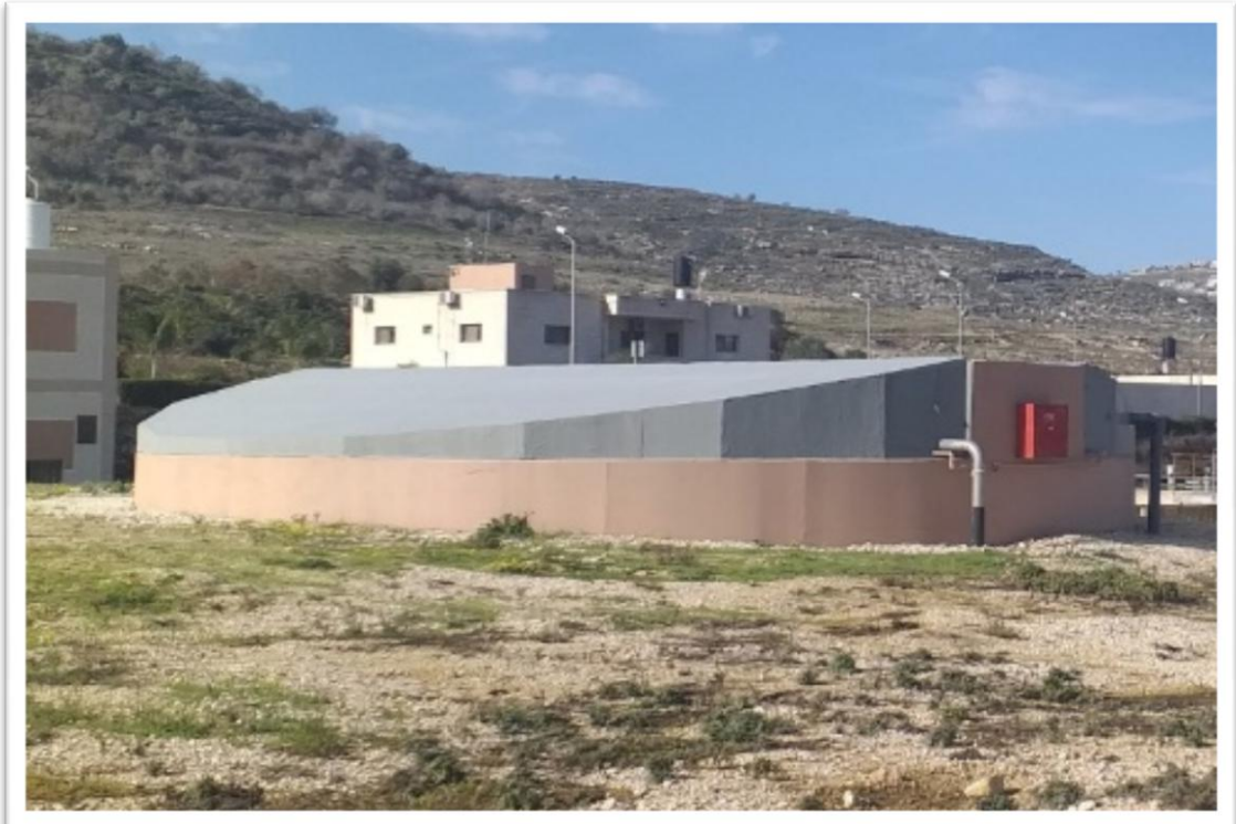
Figure (11): Covering of the primary thickener tank ( new structure design is being implemented)
