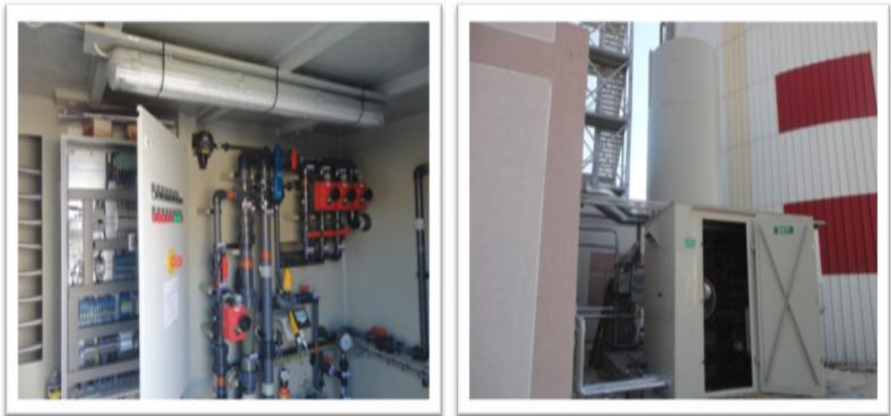
Figure (21): Nablus West desulfurization unit
