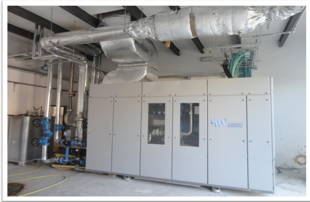
Figure (22): Nablus West CHP engine.
