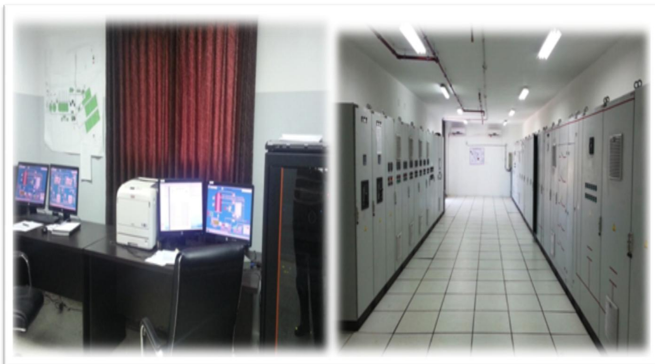
Figure (13): Nablus WWTP SCADA system
