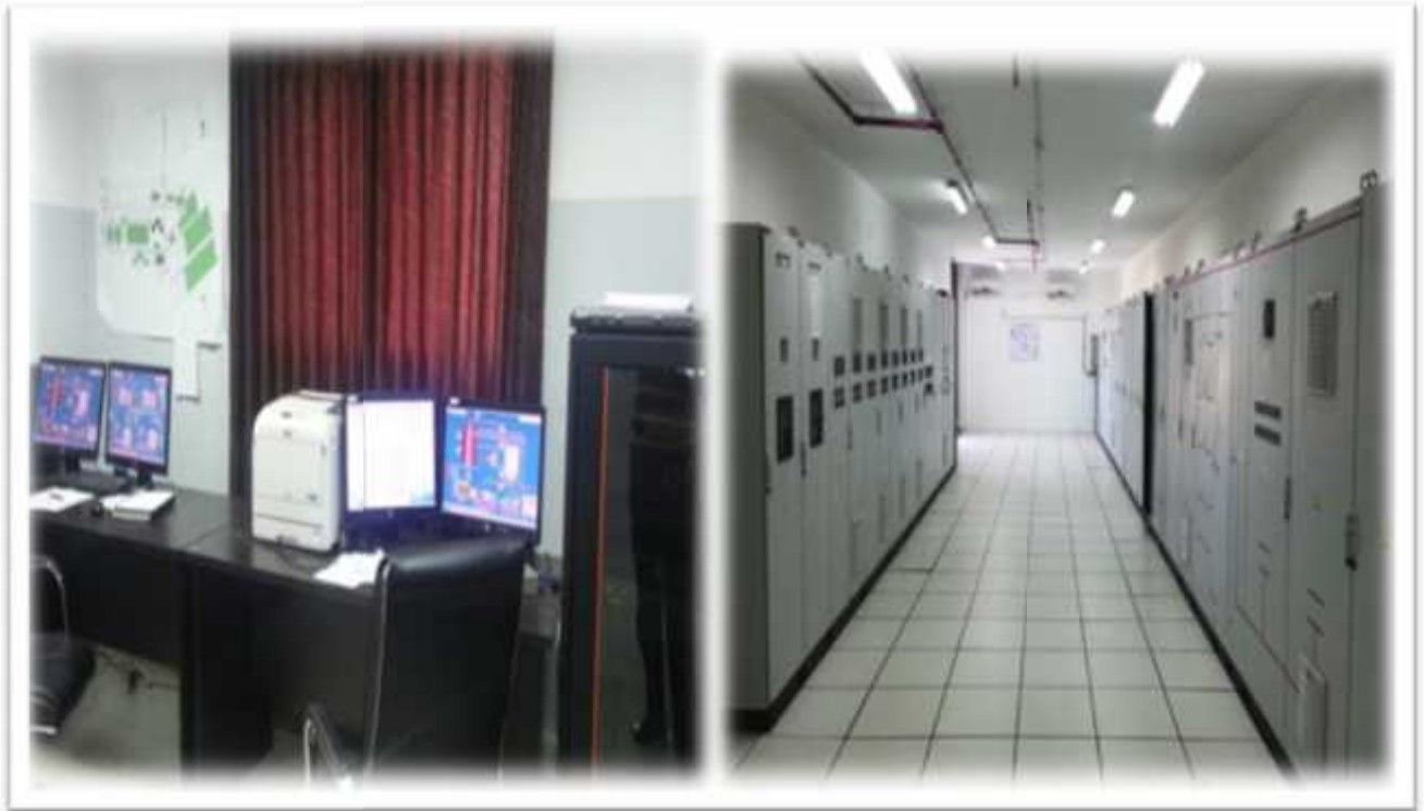
Figure (14): Nablus WWTP SCADA system
