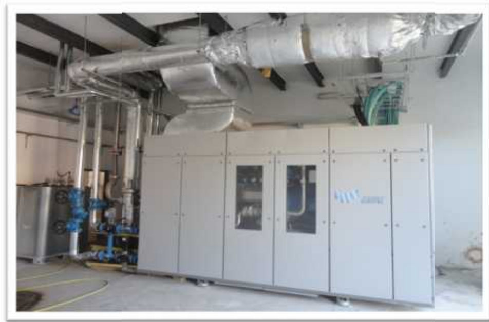
Figure (21): Nablus West CHP engine.
