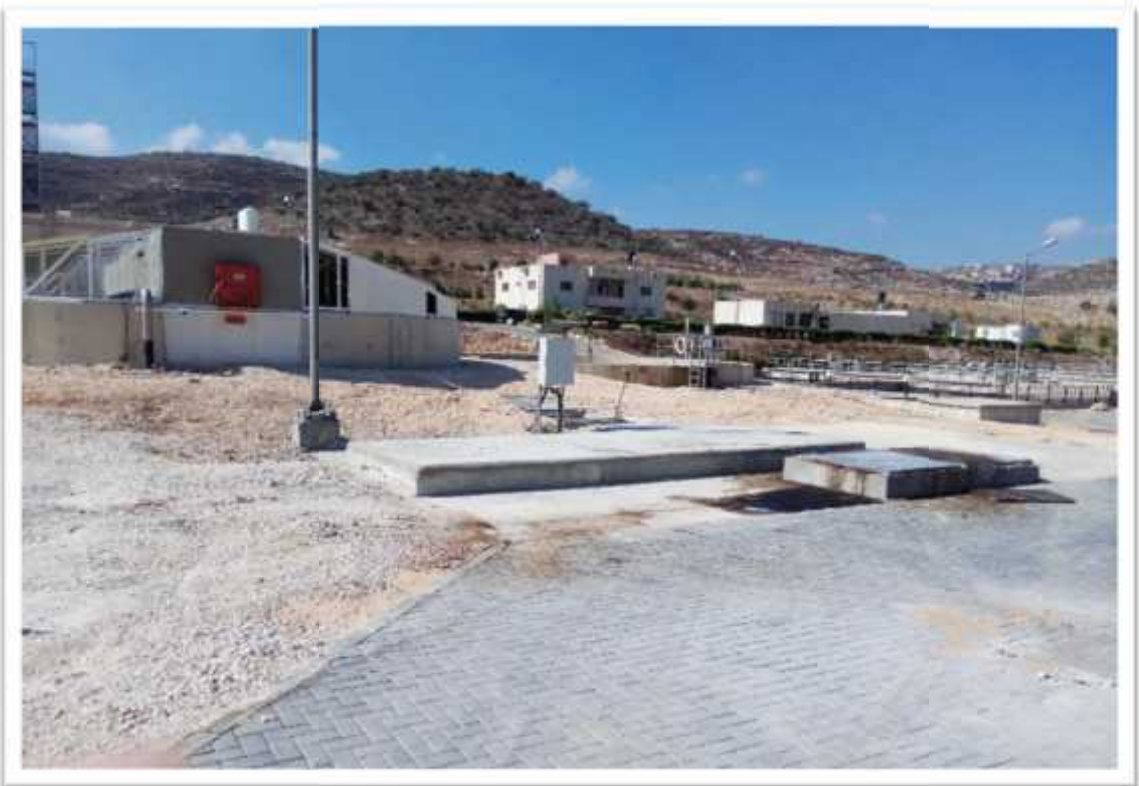
Figure (9): Storage tank of olive mill wastewater
